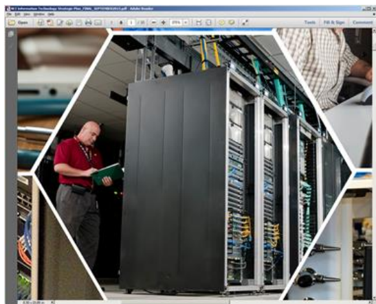
Figure 2. FNL/NCI at Frederick Data Center facilities.
