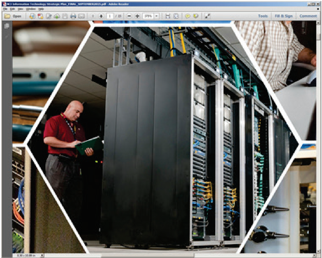
Figure 2. FNL/NCI at Frederick Data Center facilities.
