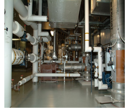
Building attic mechanical piping and exhaust infrastructure
