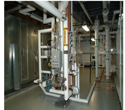
Building attic mechanical HVAC air handler infrastructure
