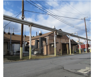
Above ground utilities
